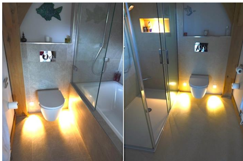
Automatic night lights in guest en-suite bathrooms
