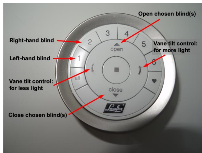
Controller for the blinds in the guest bedrooms
