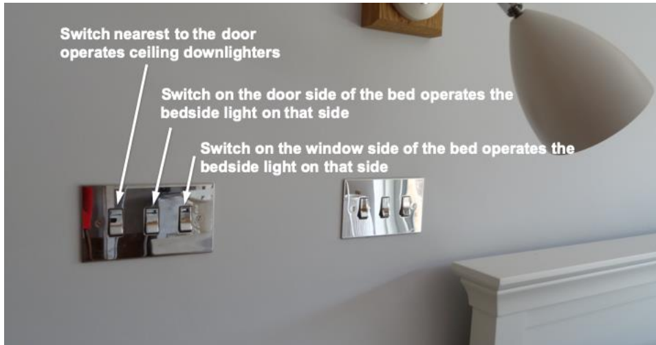
Ceiling and bedside lighting controls in guest bedrooms
